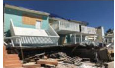
Franklin County is a coastal community, which may require special services, including beach remediation, vessel removal, and waterway debris removal.
